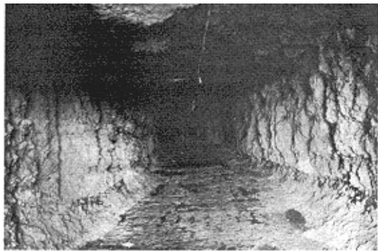
Figure 1-19. After excavation of the gravel/sand fill, protruding or loose RCC is removed. However, gallery walls are irregular and rough
