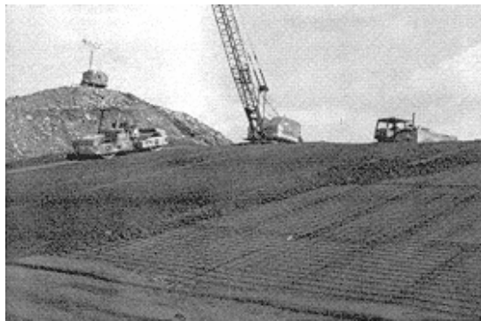
Figure 1-23. Reinforced RCC. Heavy welded wire mats can be placed in RCC to resist cracking and increase resistance to tensile stresses
